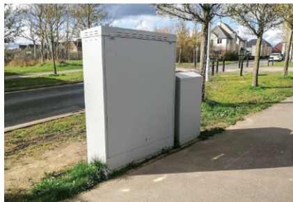
The new cabinets appearing on Love's Farm have been installed by Virgin Media
