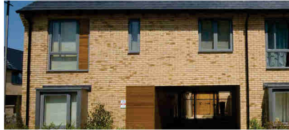
Minimal impact of rainwater goods so as not to detract from design of elevation
